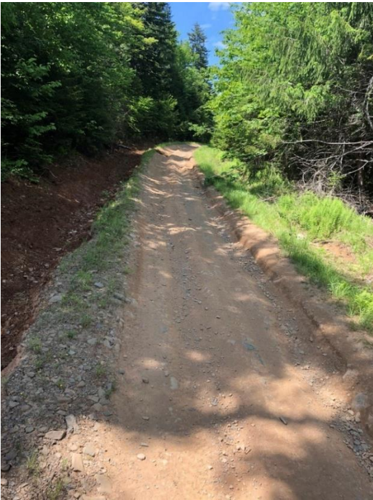
Figure 3 - $15,000 spent to repair damage done by OHVs. The ATV ruts became as deep as ditches so I had to rebuild and gravel Nicholson timber limit.
